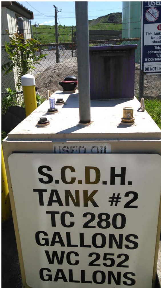
Upgraded Waste Oil Tanks at the Town of Babylon Recycling Center
